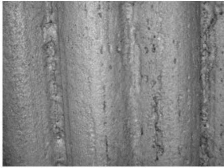
Fig. 5 Alloy 625 overlay on the waterwall revealing typical pitting type corrosion attack
