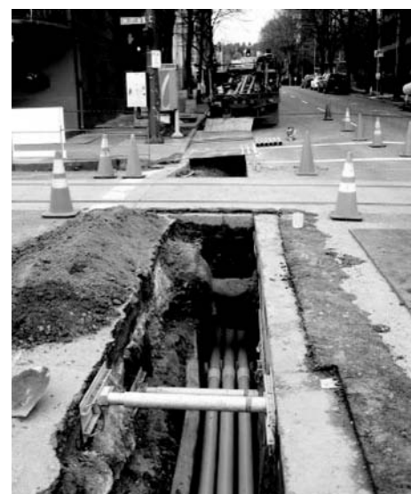
Fig. 9 Utility work at existing track slab. Tracks remain operational during excavation; however, utility work stops and moves out of the way to allow train to pass unimpeded.
