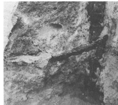
Fig. 13 Severe corrosion on reinforcing steel from the column shown in Fig. 12
