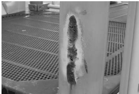
Fig. 4 Once protective coatings have been removed from playground equipment, corrosion occurs rather rapidly, accelerated by dirt, moisture, and other environmental factors including human contact. Courtesy of the NRPA NPSI
