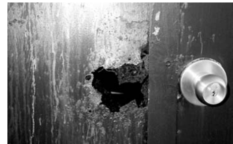
Fig. 6 Close-up of corrosion on doors shown in Fig. 5
