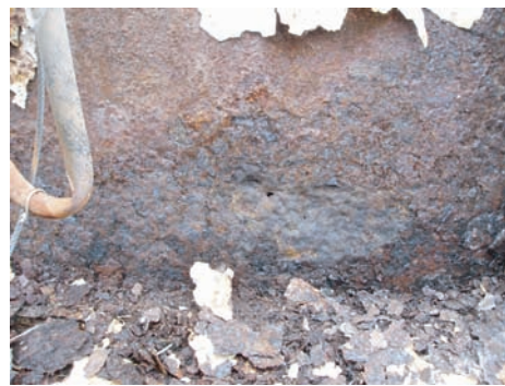
Fig. 17 Through-wall corrosion under insulation of a large coated carbon steel storage tank. Courtesy of Paul Powers, GE Inspection. See the article "Effects of Process and Environmental Variables" in this Volume.
