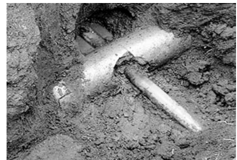
Fig. 14 Clay sewer line breached as a new gas distribution line was laid, due to lack of knowledge of where the sewer lines were located. A remote camera inserted into the sewer lines was later utilized to ascertain that no additional breaches had occurred.
