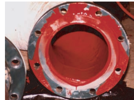
Fig. 11 In situ epoxy coating applied to the inside of the pipe shown in Fig. 10 after abrasive blast cleaning
