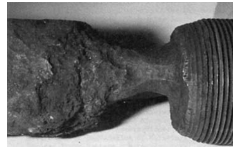
Fig. 3 Reactor coolant pump closure stud degraded by exposure to borated water. Source: Ref 20
