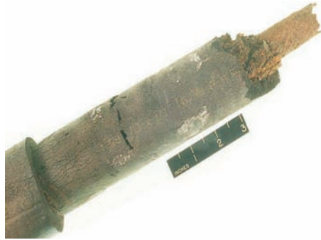
Fig. 8 Corrosion of hot water line after insulation was degraded by water intrusion
