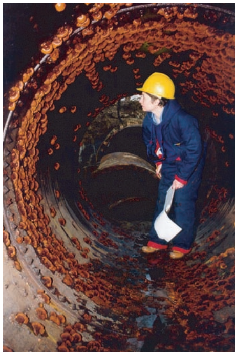
Fig. 38 A 1.5 m (60 in.) cast iron pipe with tuberculation. Courtesy of Terry Bickford. See the article "Corrosion in Potable Water Distribution and Building Systems" in this Volume.
