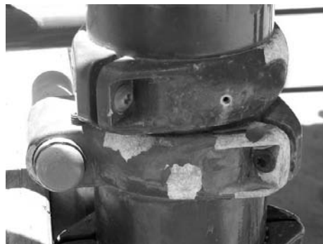
Fig. 7 White rust on galvanized parts will cause paint to blister off and provides little protection against subsequent rusting of the metal underneath. Courtesy of the PDRMA
