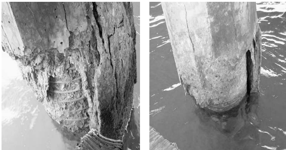
Fig. 14 Severe concrete degradation caused by rebar corrosion of piers of a NAVSTA bridge in Pearl Harbor, HI
