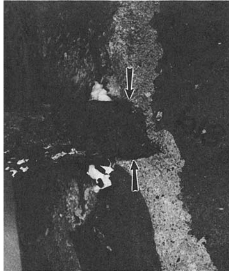
Fig. 15 Severe corrosion and cracking (arrows) on wall tie
