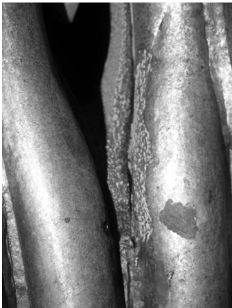
Fig. 28 Preferential corrosion of the 304L stainless steel layer in a composite tube. Corrosion occurs at the edge of the bolt-on casting in a primary air port and extends out toward the fire-side crown of the tube
