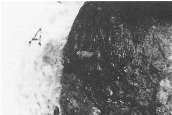
Fig. 19 Posttensioning anchorage with broken wire extending from anchor plate
