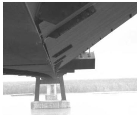
Fig. 33 Protective patina tightly adhering to weathering steel on bridge exterior
