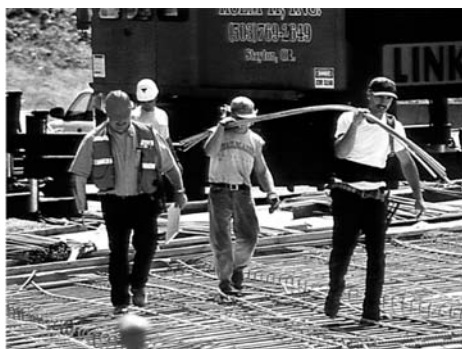
Fig. 32 Workers can walk on stainless steel bar, where they should not with epoxy-coated reinforcement.
