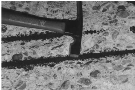
Fig. 49 Chloride ion induced rebar corrosion in a concrete splitter box that directed flow to two primary clarifiers in a bleached sulfite mill
