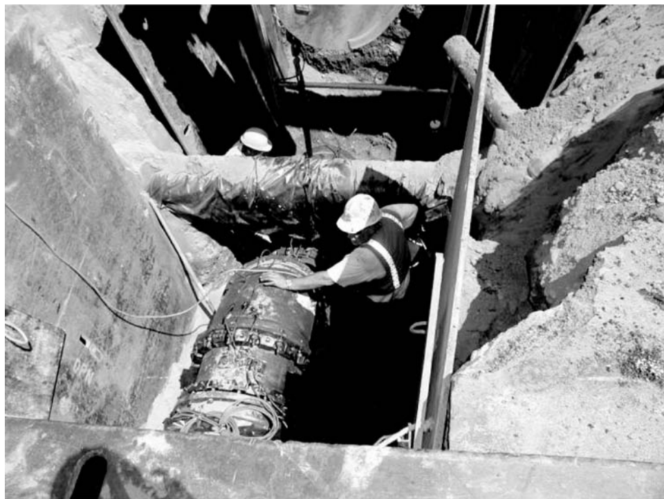
Fig. 14 Vertical offset of a 24 in. (0.6 m) ductile iron water main to accommodate an existing 12 in. (0.3 m) main.
