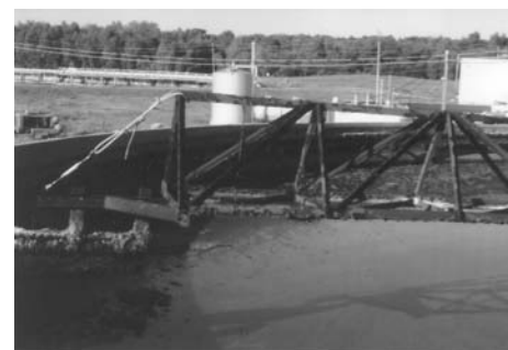
Fig. 46 Badly corroded rake mechanism in a primary clarifier
