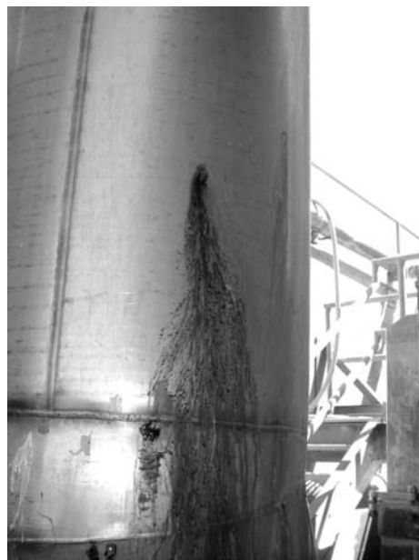
Fig. 45 Resultant leak of 316L stainless steel due to internal SRB activity
