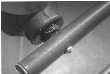
Fig. 6 A noncompatible metal bushing in contact with a stainless steel bolt and other adjacent metal surfaces if left uncorrected may corrode away and weaken the connection. Courtesy of the NRPA NPSI
