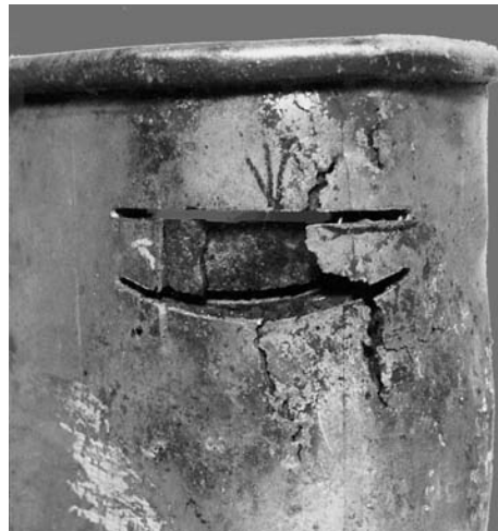
Fig. 27 Galvanic corrosion between a T439 outer muffler wrap and inner T409 shell caused corrosion debris to build up between the layers and split the outer wrap. Crack visible in wrap despite section removal to show corrosion debris
