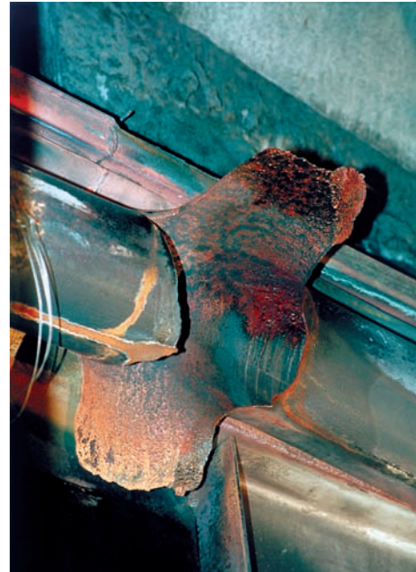
Fig. 32 Feedwater pipe thinning and rupture. See the article "Corrosion of Steam- and Water-Side of Boilers" in this Volume.
