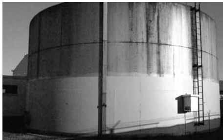
Fig. 12 Deluge tank (for fire-suppression system) with test patches overcoat applied to lower half of exterior surface. Later, the entire tank was overcoated with a moisture-cure polyurethane system
