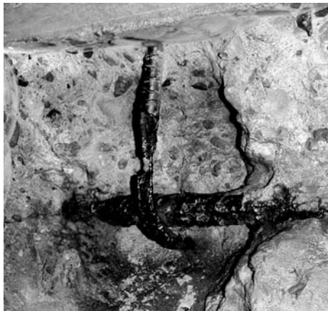
Fig. 14 Closeup of a fully failed pile cap stirrup. Note that immediately above the severely corroded area, the bar shows no sign of corrosion. The upper area was in a passive condition and served as the cathode for corrosion of the area just below. Close interval mapping of reinforcement corrosion potential can identify these situations.
