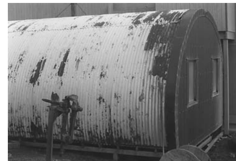
Fig. 3 Corrosion on a metal building in Antarctica. Corrosion is also evident on the steel vise. Source: Ref 12
