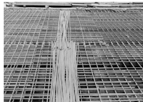
Fig. 27 Epoxy-coated reinforcement (ECR) loosely stacked on in-place ECR
