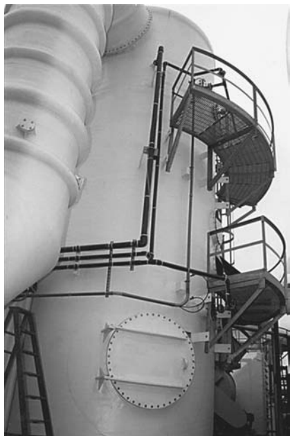
Fig. 6 A scrubber tower constructed with fiberglass. Courtesy of Branch Environmental Corporation
