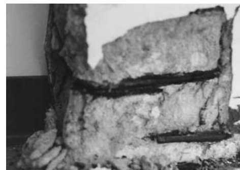
Fig. 4 Spalling on precast concrete panels occurred in three years after exposure to seawater during shipment. Reinforcing bars are exposed.
