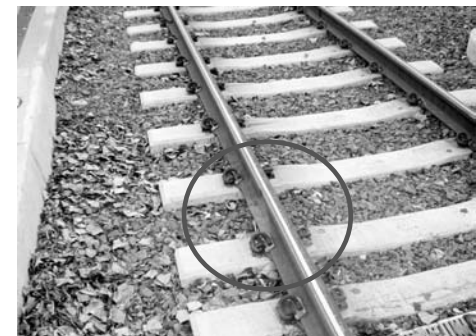
Fig. 3 Insulated tie-and-ballast track with concrete ties and insulated clips. The ballast rock is clean and well-drained; however, leaves are accumulating.
