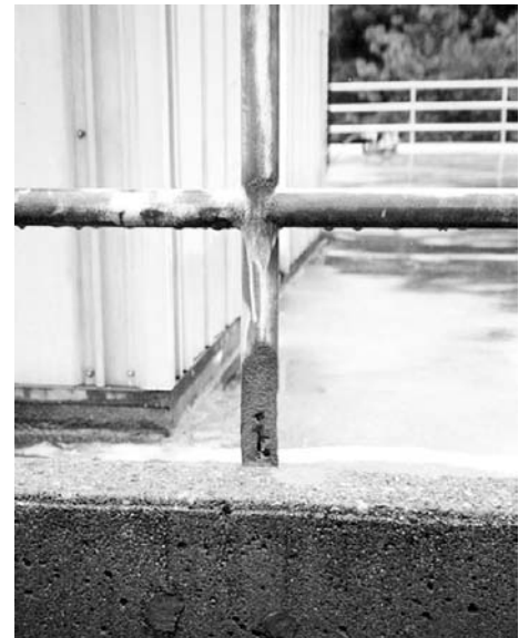
Fig. 3 Corrosion pattern on a mild steel pedestrian guardrail at a military installation exposed to a coastal atmosphere
