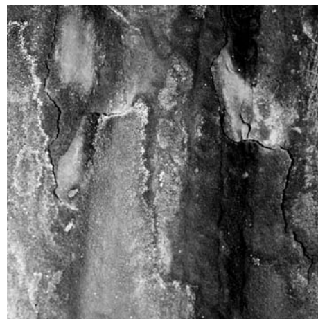
Fig. 26 Spalling of a plasma sprayed coating as a result of poor surface preparation prior to the application of the coating
