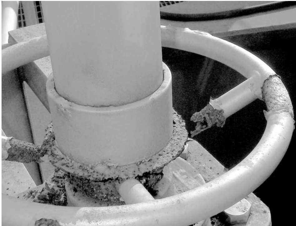
Fig. 9 Corroded control handle exposed to corrosive atmosphere at a wastewater treatment plant on a military installation
