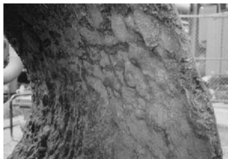
Fig. 44 Typical carbon steel corrosion morphology due to SRB action
