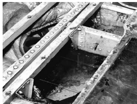
Fig. 11 Moisture accumulation from blocked drain
