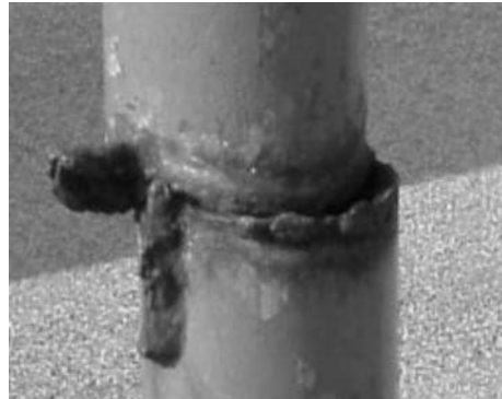
Fig. 5 If a weld joint separates as a result of corrosion, it is difficult to repair to its original structural integrity. Courtesy of the NRPA NPSI
