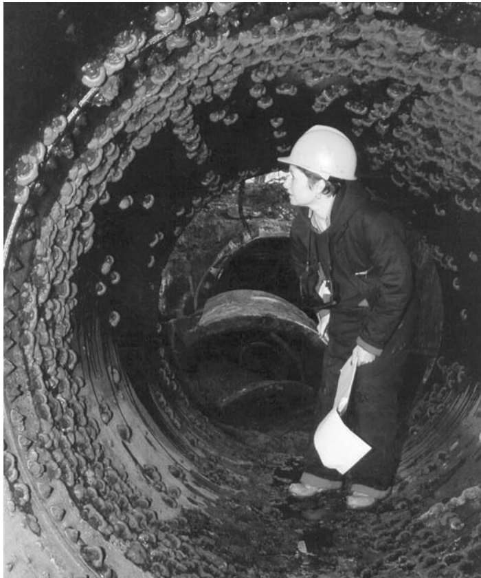
Fig. 2 A 1.5 m (60 in.) cast iron pipe with tuberculation. Courtesy of Terry Bickford
