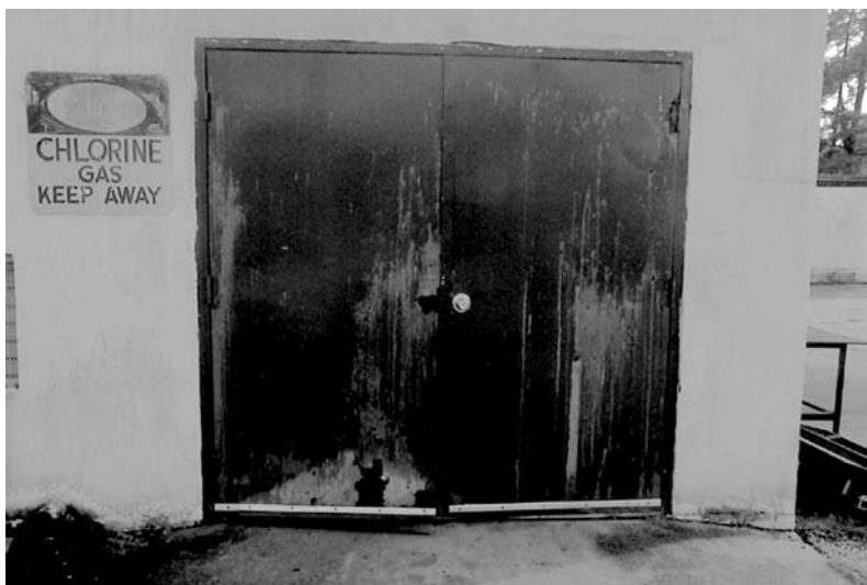
Fig. 5 Corroded metallic doorway at a military installation water treatment plant due to chlorine atmosphere
