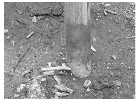
Fig. 8 Galvanized post at a concrete footer corrodes from a moist subgrade environment. Chlorides from the fresh concrete can accelerate the corrosion process. Courtesy of the PDRMA
