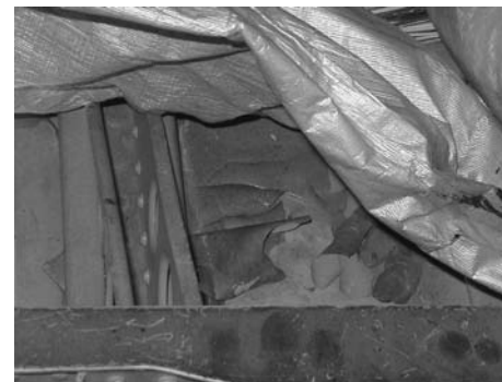
Fig. 18 Loss of paint adhesion caused by silicone contamination
