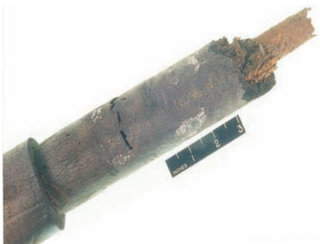
Fig. 16 Corrosion of hot water line after insulation was degraded by water intrusion. See the article "Corrosion Control for Military Facilities" in this Volume.
