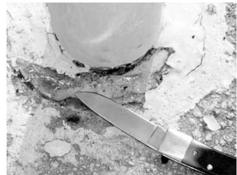
Fig. 4 Close-up of the base of the vertical pole shown in Fig. 3. Note that the pole was soldered in place using a lead-base low-melting-point alloy.
