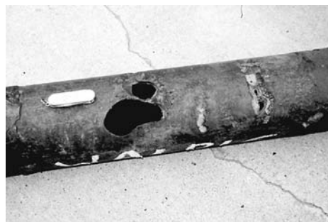
Fig. 5 Pipeline that experienced stray current corrosion caused by inverting the electrical leads to a cathodic protection rectifier
