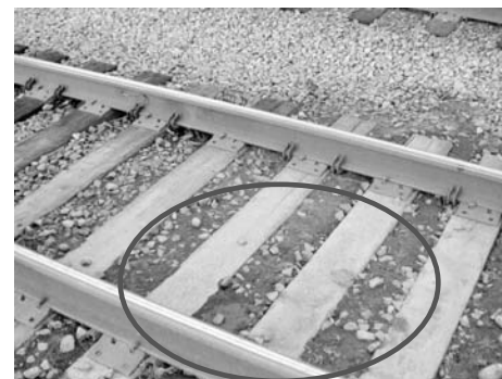
Fig. 2 Noninsulated tie-and-ballast, with wooden ties, metal spikes, and ballast rock that is fouled with soil fines and moss
