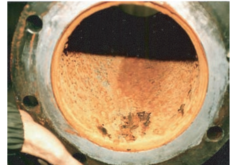
Fig. 10 Corroded water pipe contaminates water that services an Air Force Base hospital
