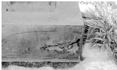
Fig. 2 Close-up of corrosion at the base of the pole shown in Fig. 1
