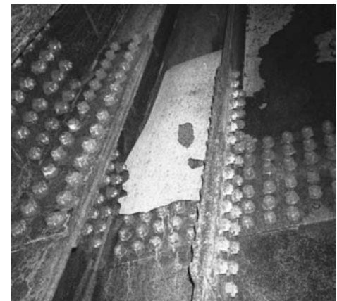
Fig. 34 Wallpaper-like corrosion product peeling from weathering steel on bridge interior
