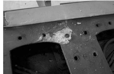
Fig. 14 Galvanic corrosion of an F/A-18 aircraft wing substructure resulting from composite doors attached to aluminum substructure with titanium and steel fasteners in the presence of moisture. Courtesy of S. Long, Naval Air Depot—North Island
