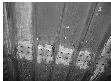
Fig. 9 Exfoliation corrosion of a integral fuel tank on a P-3 aircraft resulting from long-term exposure to moisture, salts, and fuel-system icing inhibitors. Courtesy of J. Benfer, Naval Air Depot—Jacksonville
