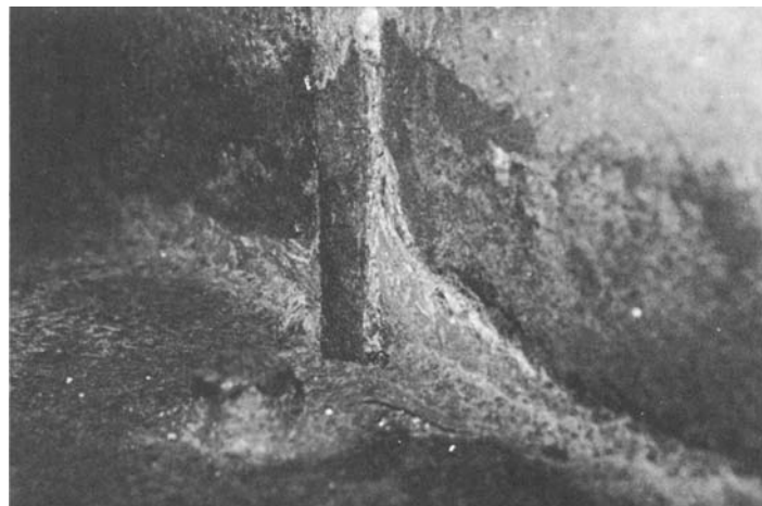
Fig. 9 Heavy buildup of corrosion scale on weathering steel structural members in conditions of poor air circulation, high humidity, and no wetting/drying
